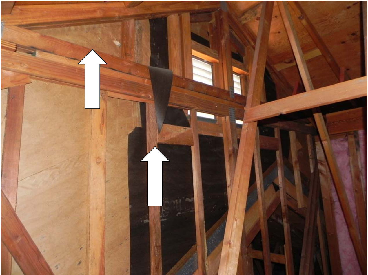
Attic Space – Gable at West End – Moisture Barrier Paper – Visible water damage and mold growth – Note: Different types and installation of moisture barrier paper
