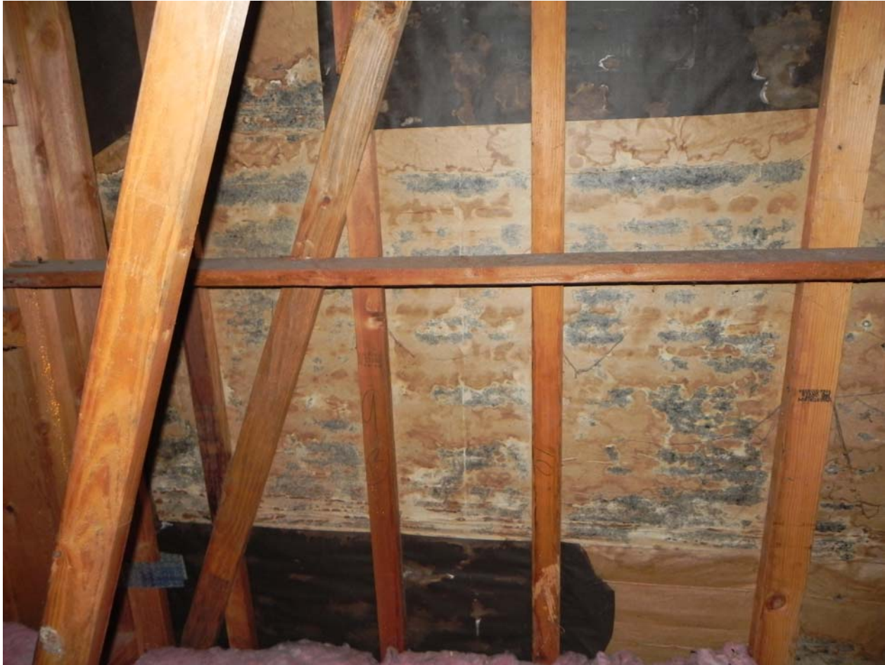
Attic Space – Gable at East End – Moisture Barrier Paper – Visible water and mold damage
