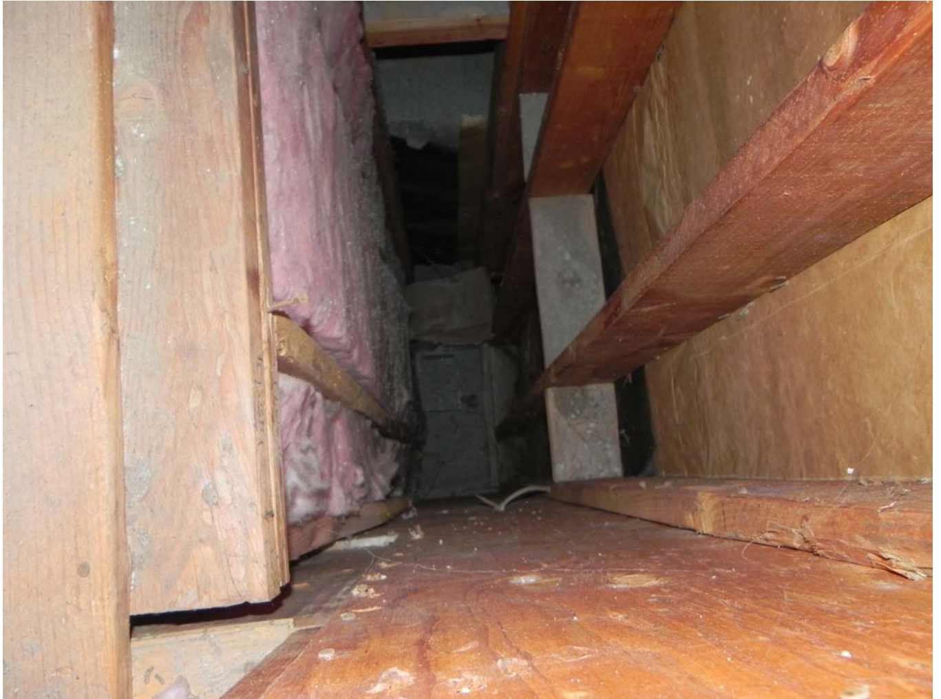
Attic Space – Chase at center of attic adjacent to the pitched roof line
