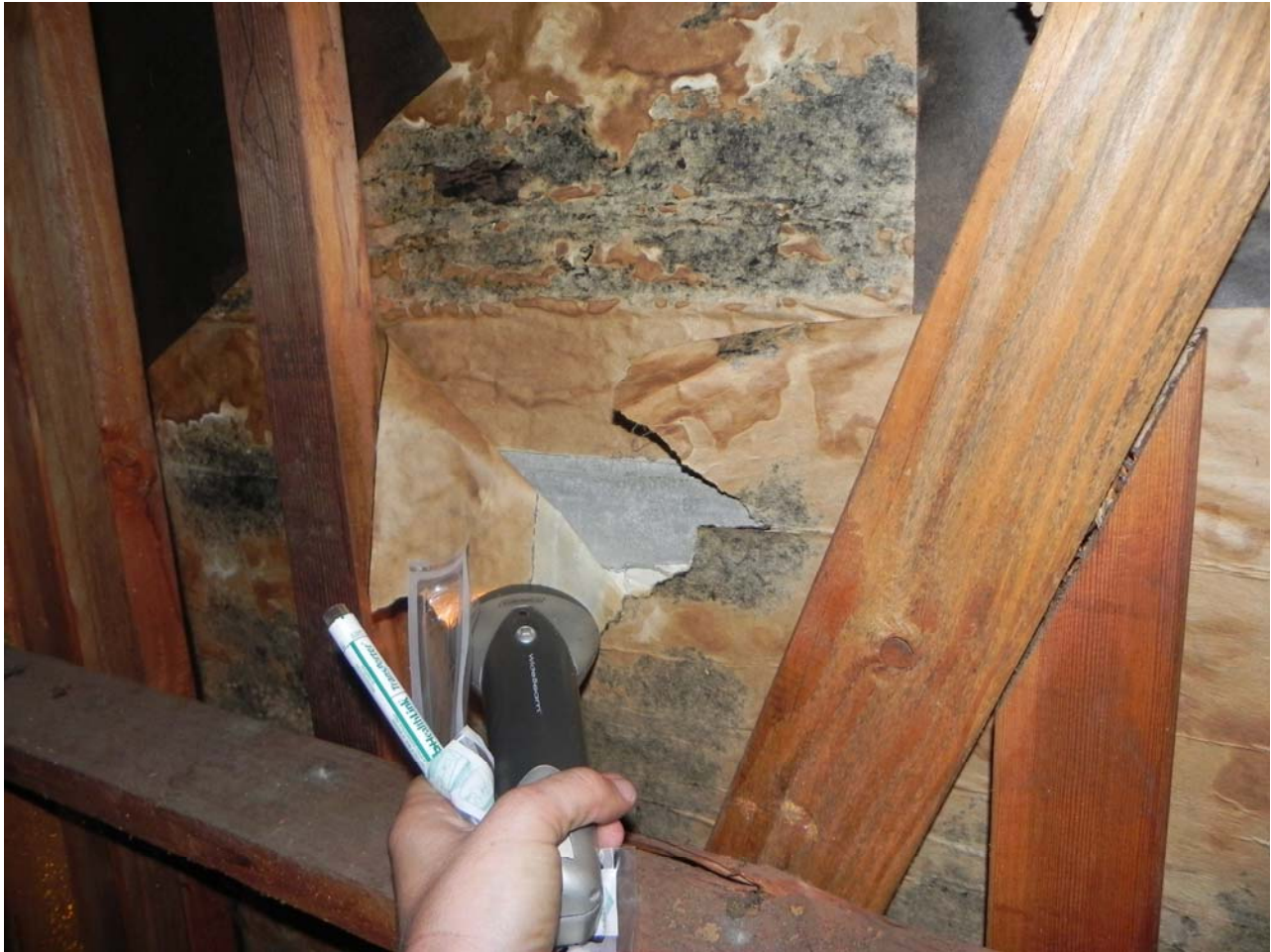
Attic Space – Gable at West End – Moisture Barrier Paper - No metal lath or substrate – Stucco applied directly to paper
