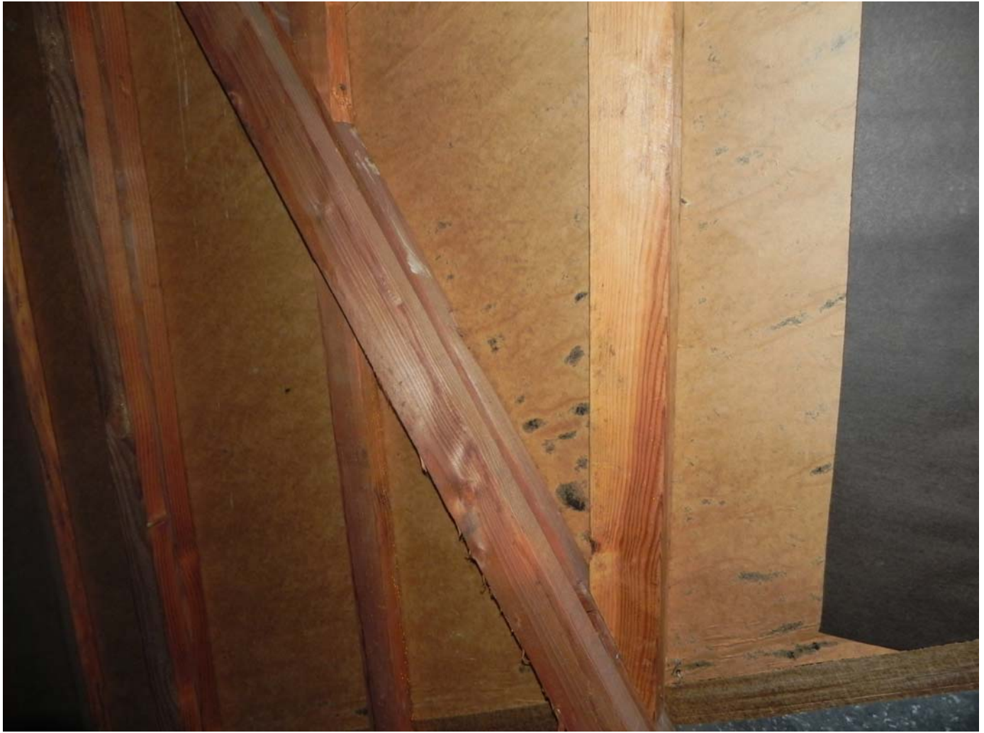
Attic Space – Gable at West End – Moisture Barrier Paper – Visible water damage and mold growth
