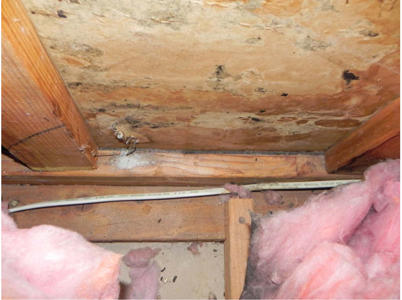
Attic Space – Gable at East End – Moisture Barrier Paper – Visible water and mold damage extending upward from attic floor
