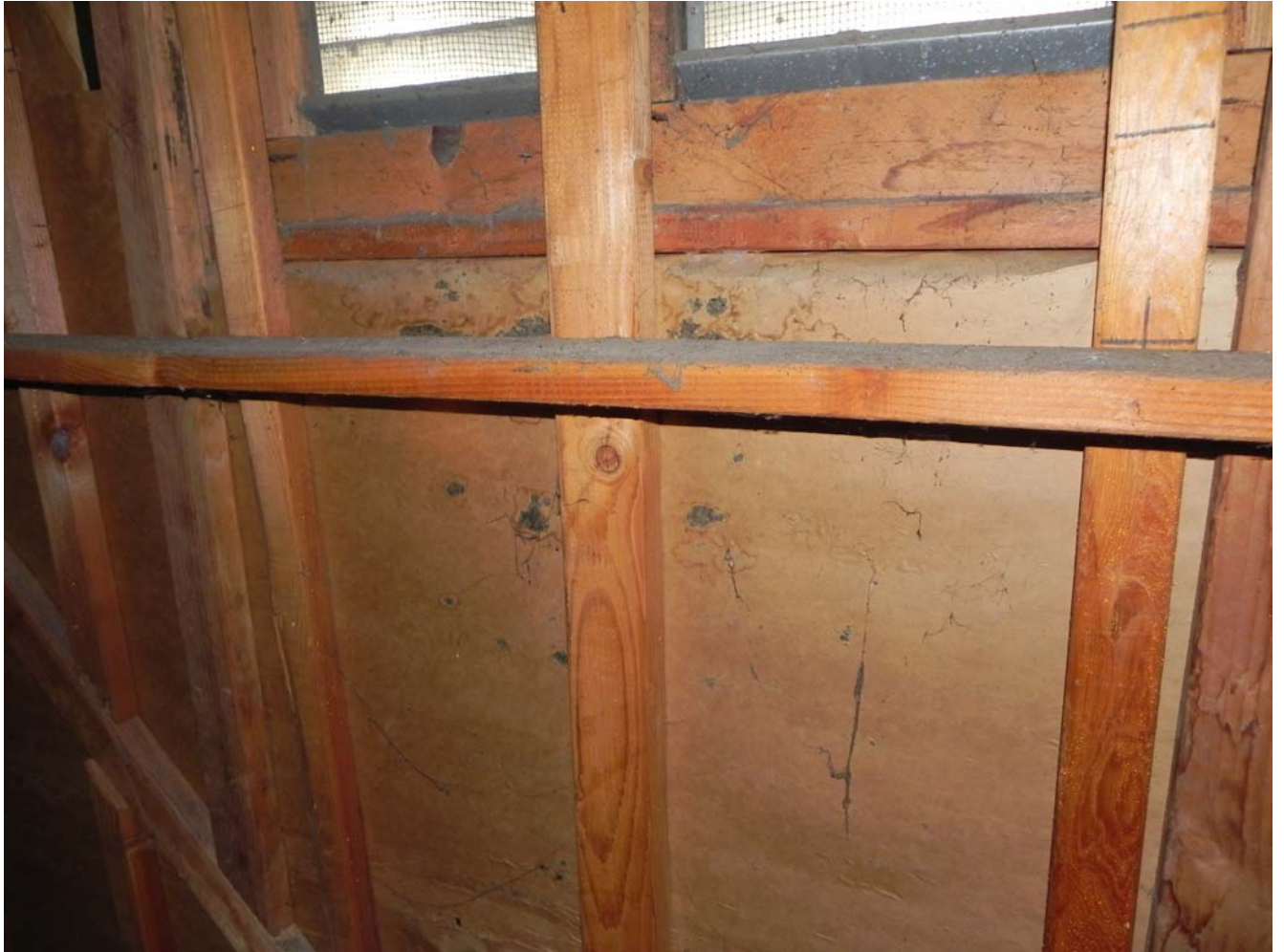
Attic Space – Gable at West End – Moisture Barrier Paper – Visible water damage and mold growth
