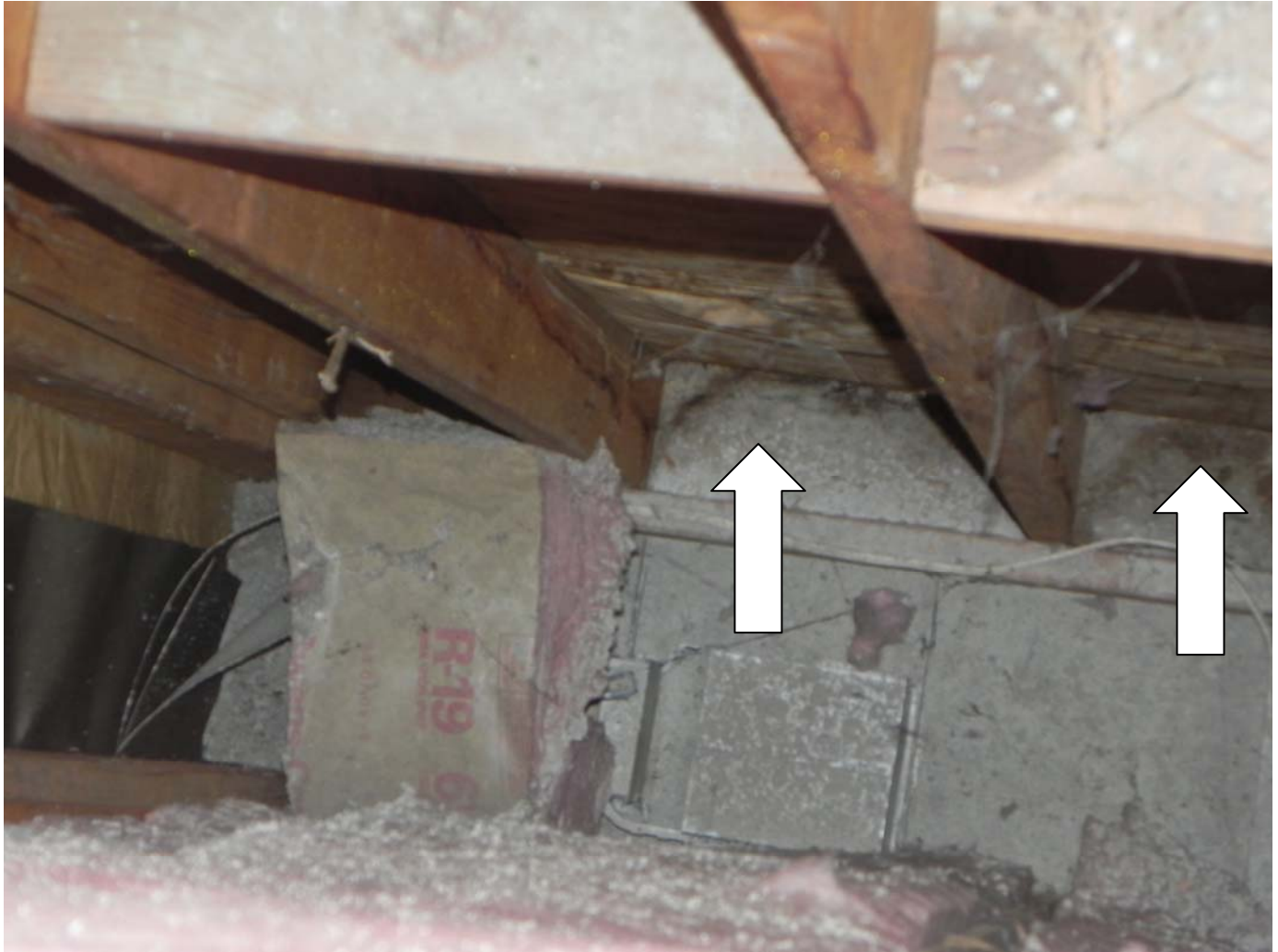
Attic Space – Chase – Center of attic – Bottom of west exterior wall (common to the garage) – Moisture barrier paper – Visible water damage and mold growth
