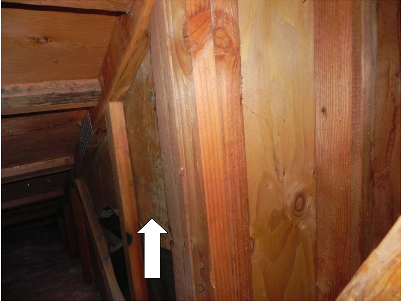
Attic Space – Gable at West End – Moisture Barrier Paper – Visible water damage and mold growth
