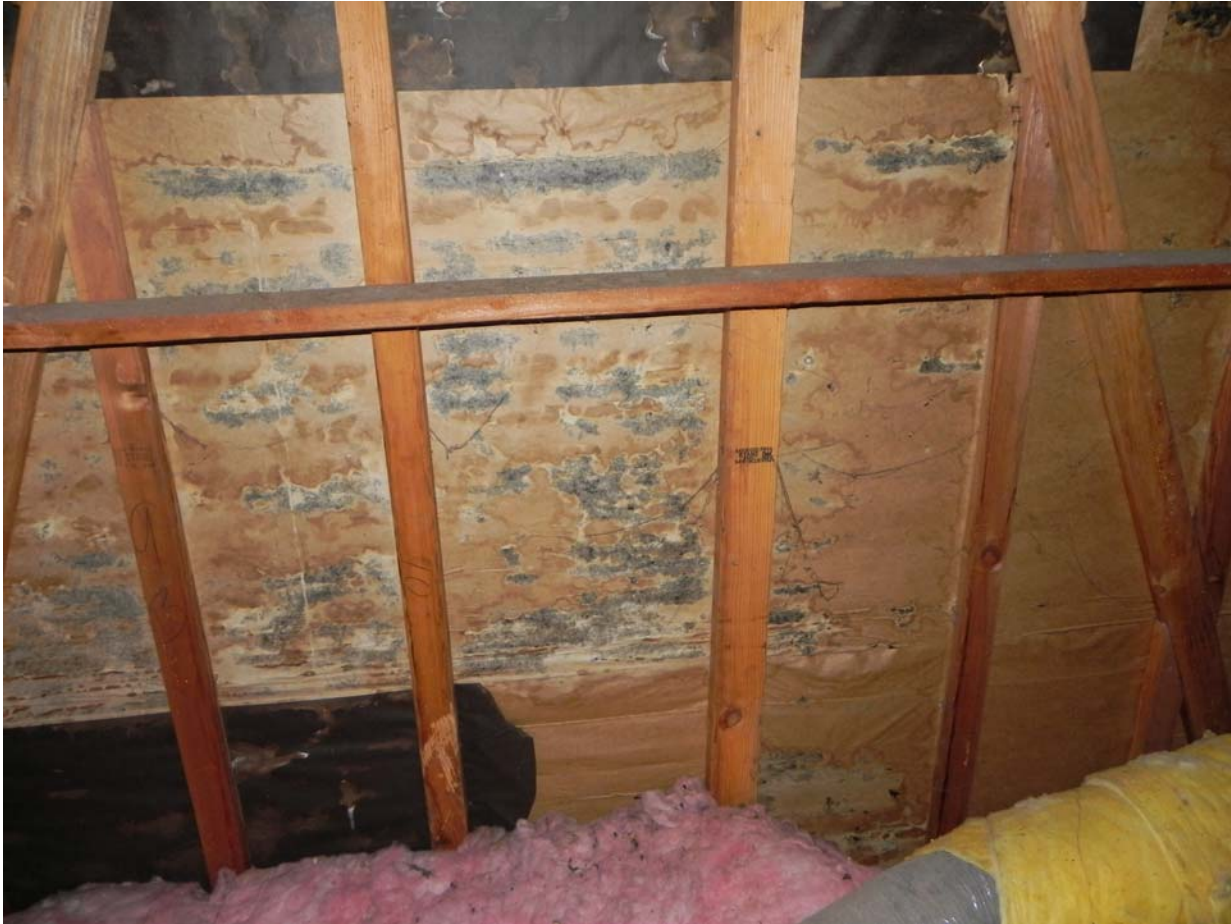
Attic Space – Gable at East End – Moisture Barrier Paper – Visible water and mold damage
