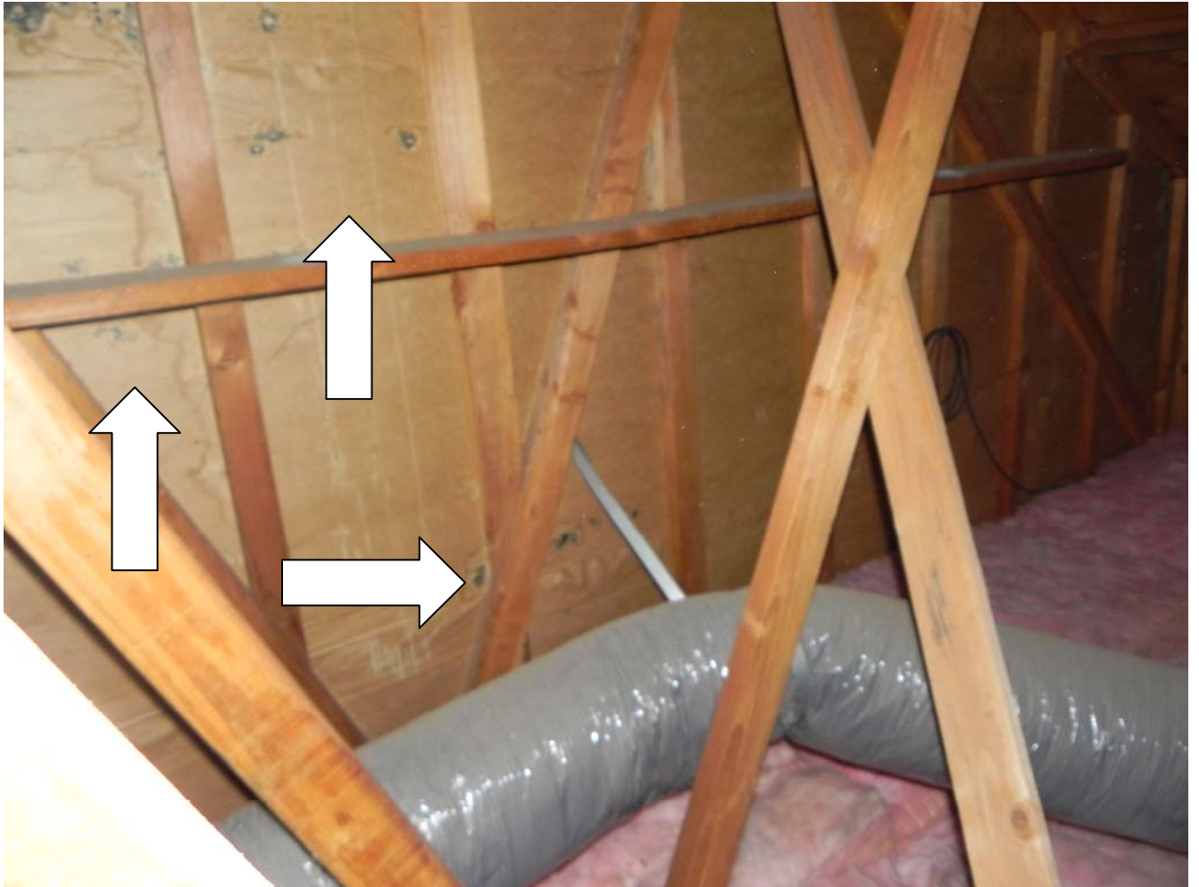
Attic Space – Gable at East End – Moisture Barrier Paper – Visible water and mold damage
